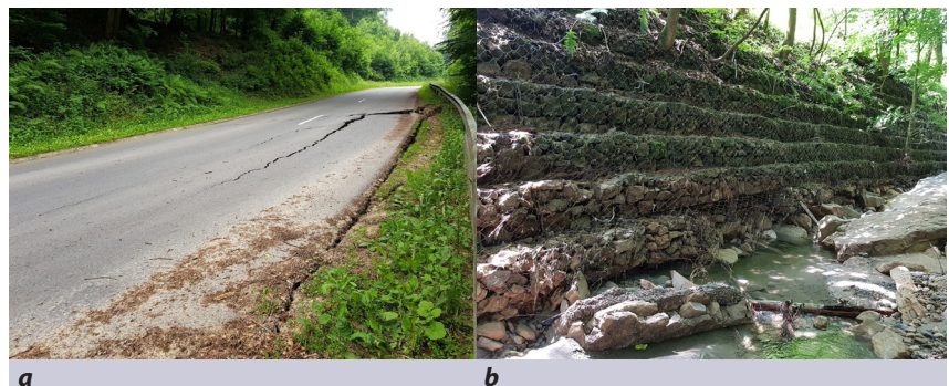
Figure 3: Examples of damage: cracks on the road (a); damaged gabion retaining wall (b).
